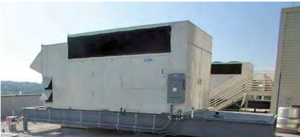
Air Handling Unit
