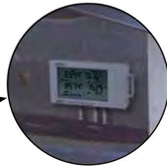
There's good mixing here, just before the inlet to the supply fan.
