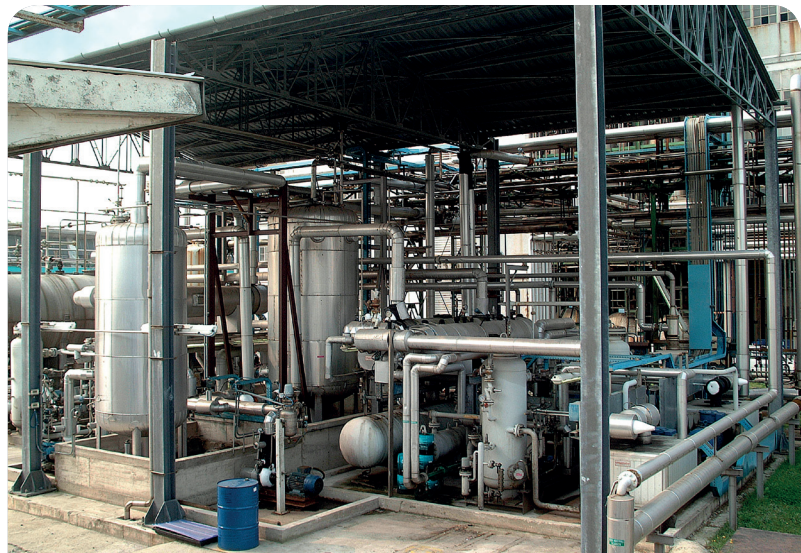
Refrigeration system for the production of antibiotics
