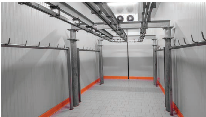
Cold Room and Storage
